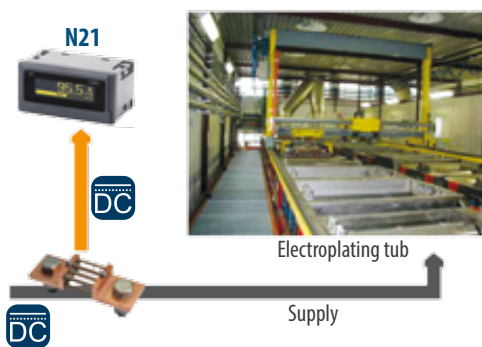
Current measurement in an electroplating plant
